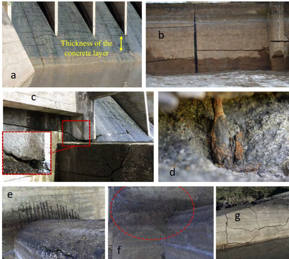
Figure 3.19: Observed damages: (a) cracks in downstream face, (b) crack of upstream face, (c) cracks of strainway and loos of concrete, (d) corrosion of rebars, (e) erosion in diaphragm, (f) cracks in diaphragms, and (g) map cracking in the retaining walls of the dike; Blanco et al. (2018)
