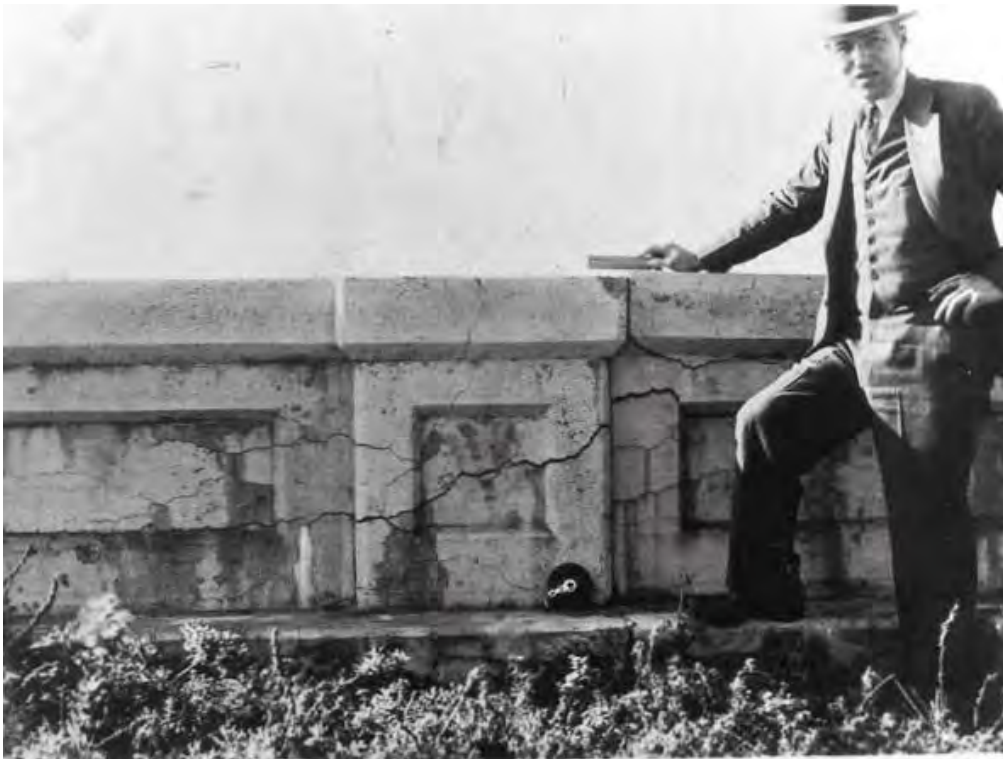
Figure 3.208. Figure 1. Thomas Stanton of the California State Division of Highways and a Bridge Parapet Wall that is Showing Signs of Damage due to Alkali-Silica Reaction. From Alkali-Aggregate Reactivity (AAR) Fact Book ; (FHWA, 2013)
