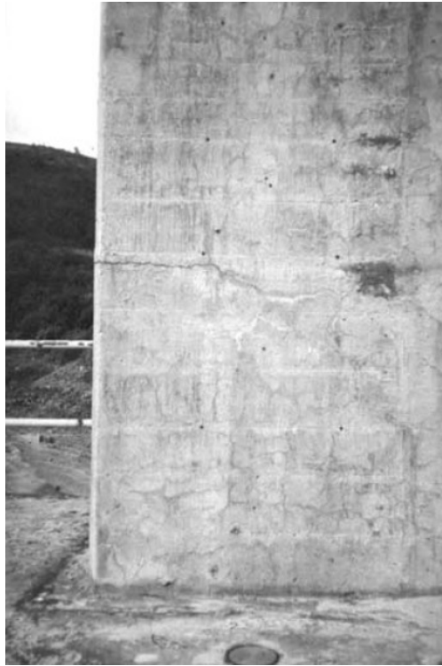
Figure 3.114: Map-like fissures on a concrete wall in the Belesar Dam; Herrador, Martínez-Abella, and Dopico (2008)
