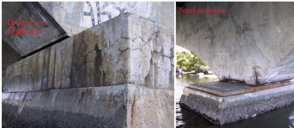
Figure 3.111: Signs of deterioration at the Paulo Guerra Bridge (left); severe steel corrosion (right); Helene, Carvalho, and Pacheco (2017)
