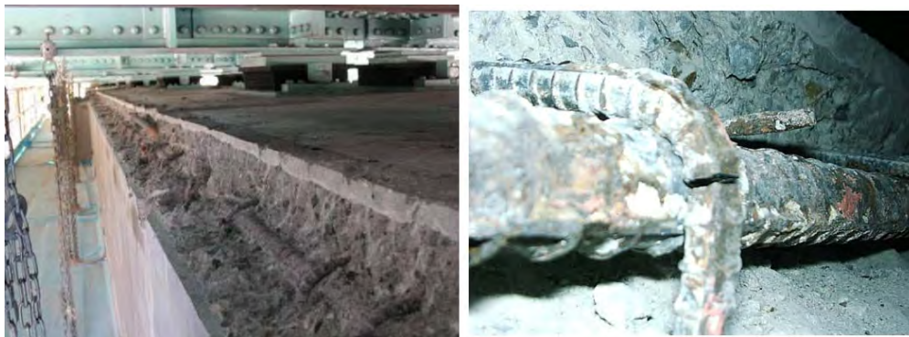
Figure 3.146: Chipping inspection of pier beam (left); Fractured steel bar (right); Miyagawa et al. (2006)
