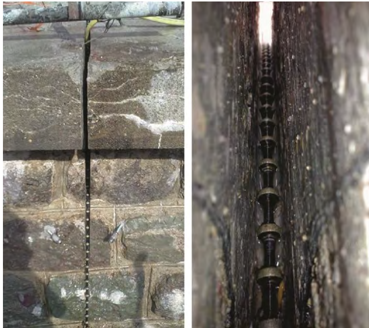
Figure 3.196: The slot cutting from downstream face. On the left, the kerb of the crest; on the right, the wire in the middle of the cutting; Sbarigia, Zinetti, and Hernandez-Bagaglia (2016)
