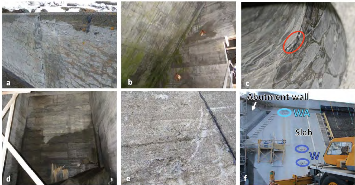
Figure 3.175: Photos of the Votna I Dam: a) map cracking at the rail of the Dam; b) map cracking inside the slab ; c) presence of ASR gel in a bore hole; d) humidity inside the slab; e) aggregates visible on the surface; f) upstream face after drilling; Plusquellec et al. (2018)
