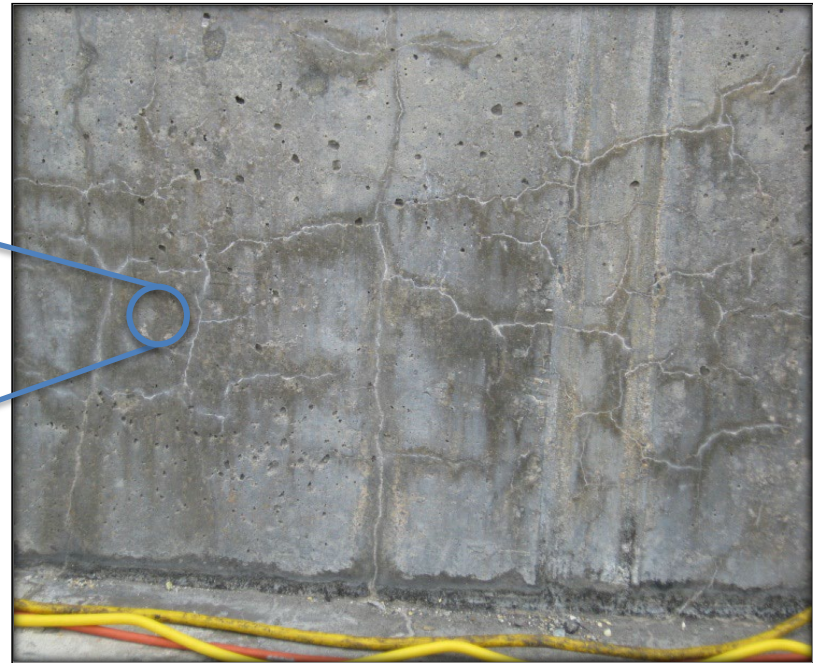
Visual signs of cracking on the surface of the concrete
