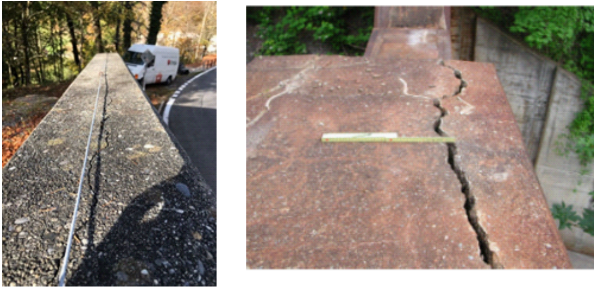
Figure 3.16: Examples of ASR driven delamination in surface reinforced concrete retaining walls in Switzerland (Courtesy Dr. Leemann, EMPA, Switzerland)
