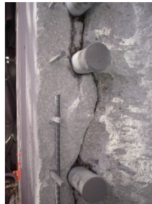
Figure 2.10: 0 Crystal River delamination (crack between the two reinforcing mats)
