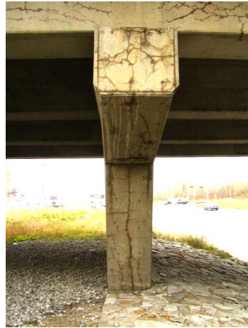
Figure 1.9: Cracking in reinforced concrete beam and column caused by ASR ( fhwa06 )
